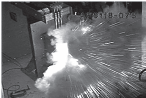
FIGURE 9.3 Simulated arc-flash incident, conducted at 250 V, 44 kA (44,000 A). Energy intensity: 8.48 cal/cm 2 .
